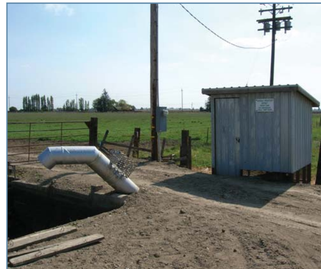
Typical Pumping Plant
