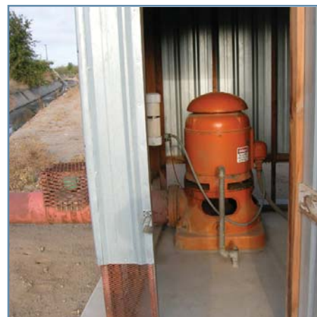
Pumping plant similar to the one shown above pumps groundwater and discharges it to the District's conveyance system.
